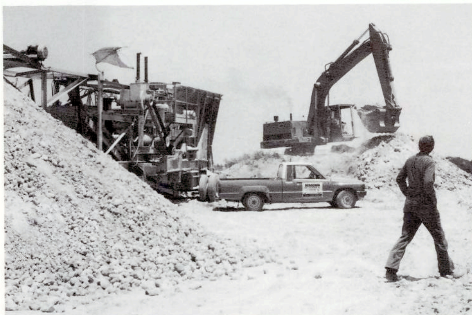
Two other Cat units help provide the crushed limerock used for the new fill. This material was dredged 4-5 years prior from canals and stockpiled. The 235 feeds the portable crusher, which in turn makes new stockpiles of the spec' rock. The 950B loader loads from these into the fleet of 12-14 yd. dump trucks hauling 5 miles to the job site.
